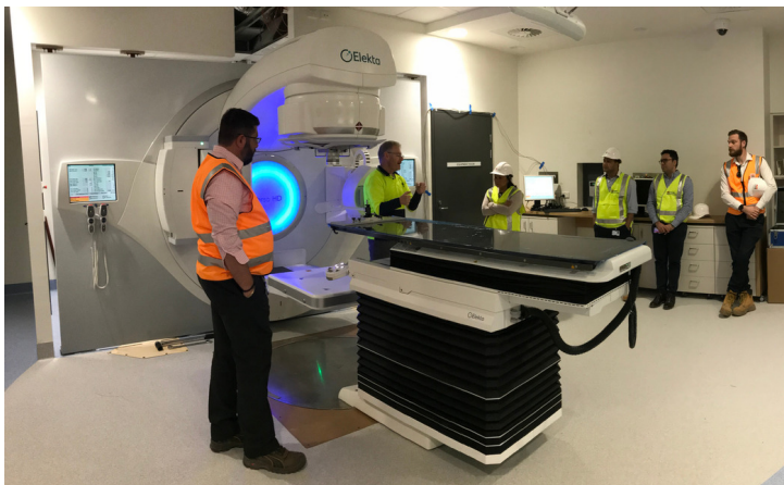
The project team is working closely with the experienced radiation therapy team at the Nepean Cancer Care Centre to commission the new linear accelerator.
